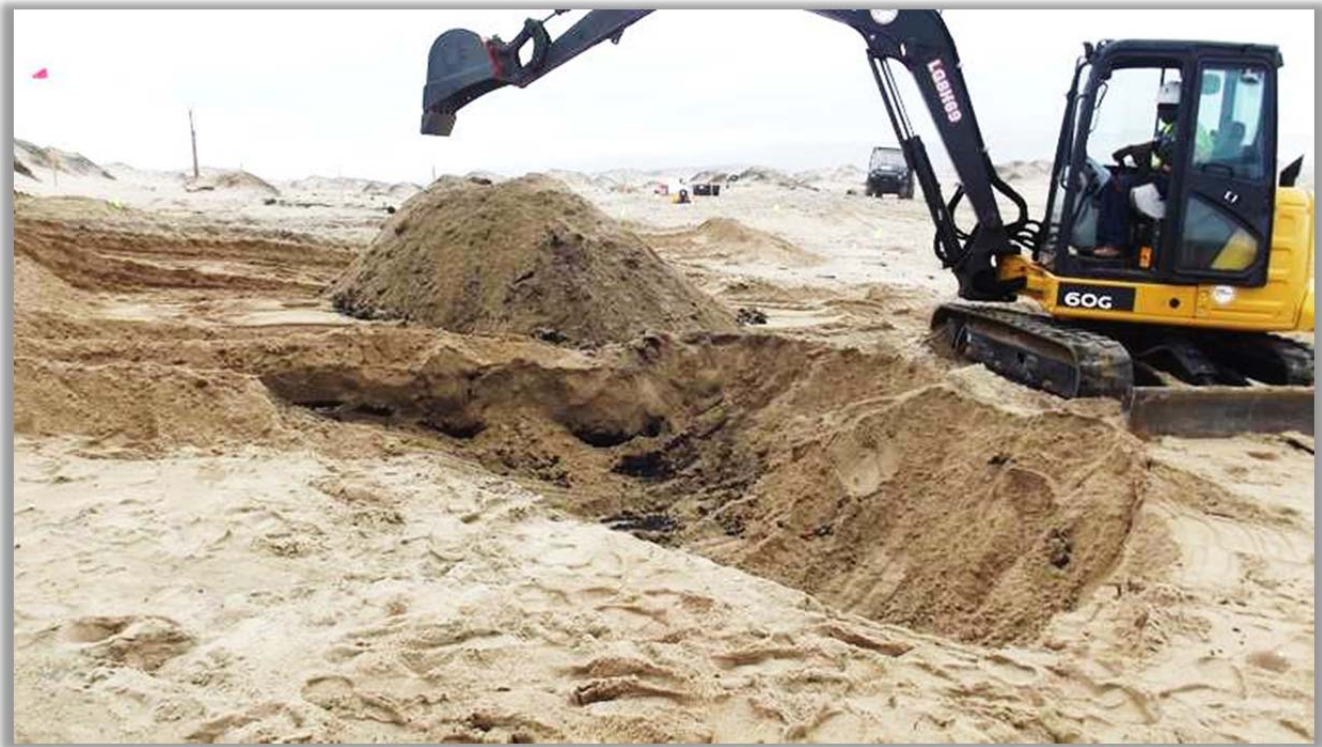
Excavating sump material. Although much of the exterior material was hard, deeper material in the interior of the sump was more pliable.
