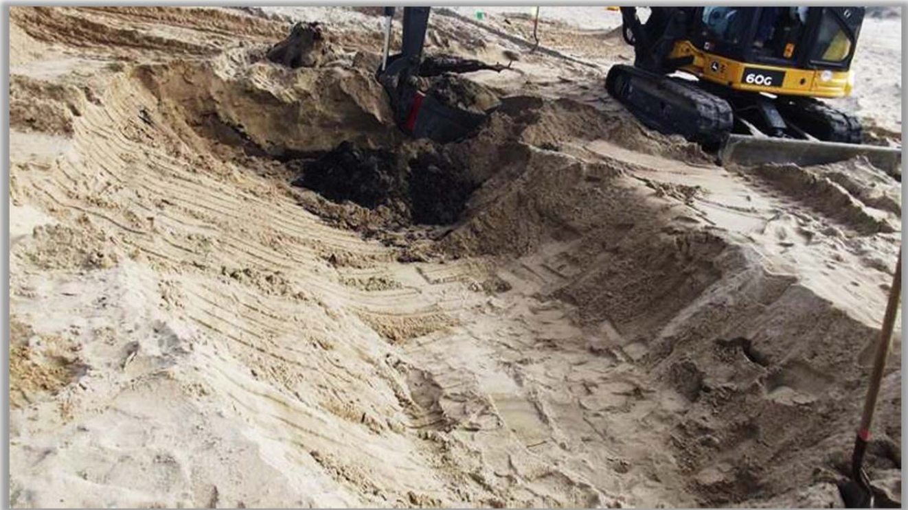
As visible in the photo above, the sump material was excavated to an approximate depth of 2-3 feet. The area was sampled and will be backfilled with clean overburden after all the sump material has been removed. Chevron anticipates at least one additional full day of excavation.
