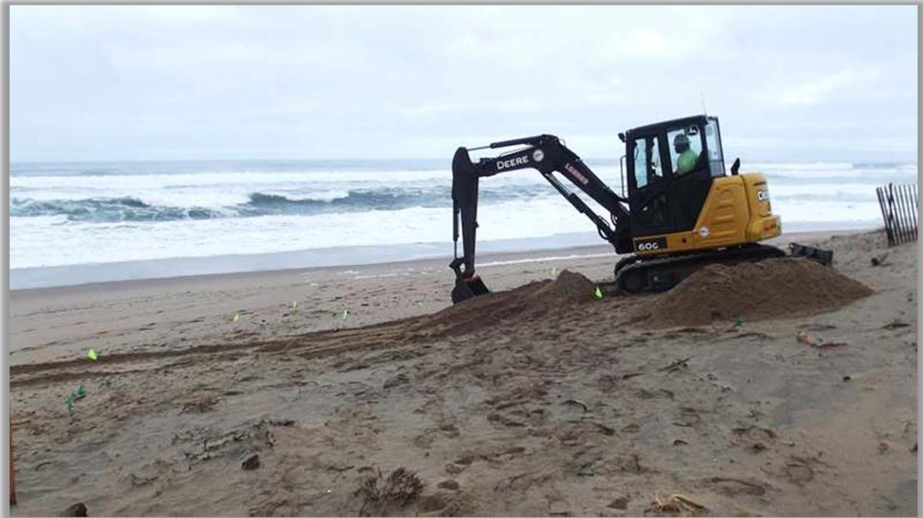
Mini-excavator used to clear clean overburden off of the sump material. This clean overburden will eventually be used to backfill over the excavation pit at the conclusion of excavation.
