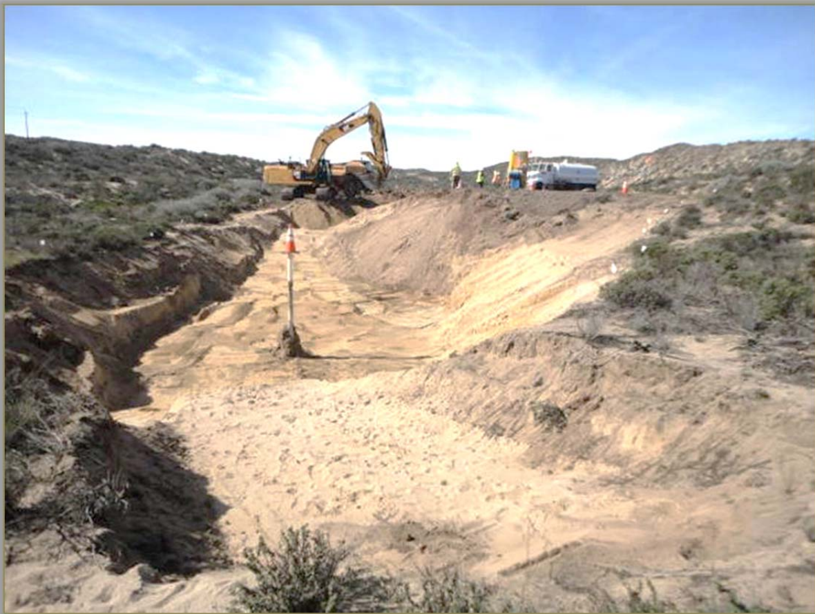
K12 Sump and Diluent Stain Removal. All of the sump material encountered in the excavation of this site was excavated; all of the diluent-contaminated soils were excavated to depths greater than four-feet deep.
