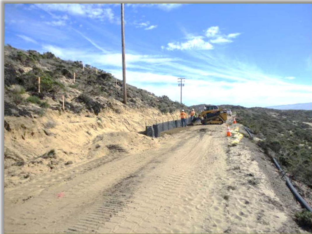
TB9 Recovery Well Road; road was widened to allow construction-related equipment safe access to the J14, I12, and I13 PROs Treatment areas. Construction team substantially reduced originally approved impacts to native habitats.
